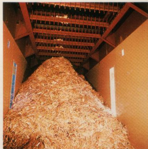
Overhead rakeback system utilizes full bin capacity.
